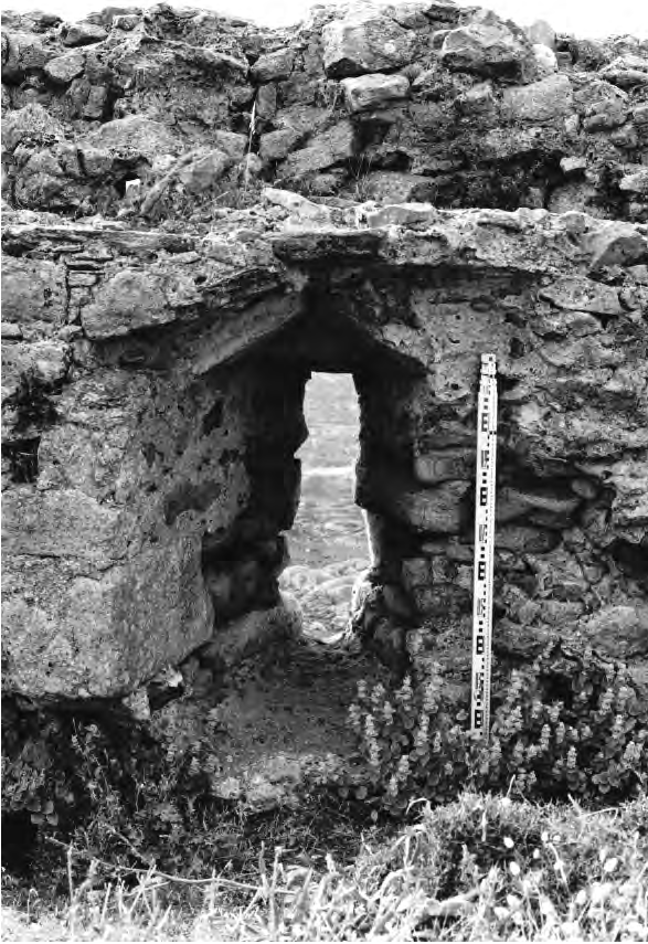
Fig. 6.17 View of a loophole from the inside of the inner defensive wall of Apano Kastro
