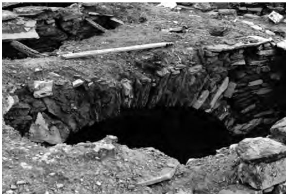
Fig. 6.99 A collapsed roof supported by an internal stone-built arch in a house at Ismaili
