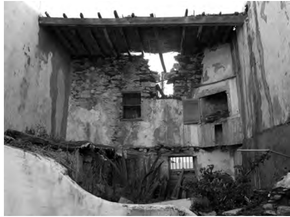
Fig. 5.40 Ruins of a broad-fronted house in the town of Naoussa, Paros
