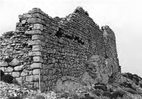
Fig. 6.25 View of Hall A from the Northeast with a long gap on the stone masonry suggesting the position of the wooden balcony-like projection
